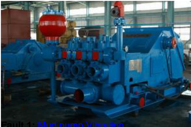
Fault 1: Mud pump Vibration
